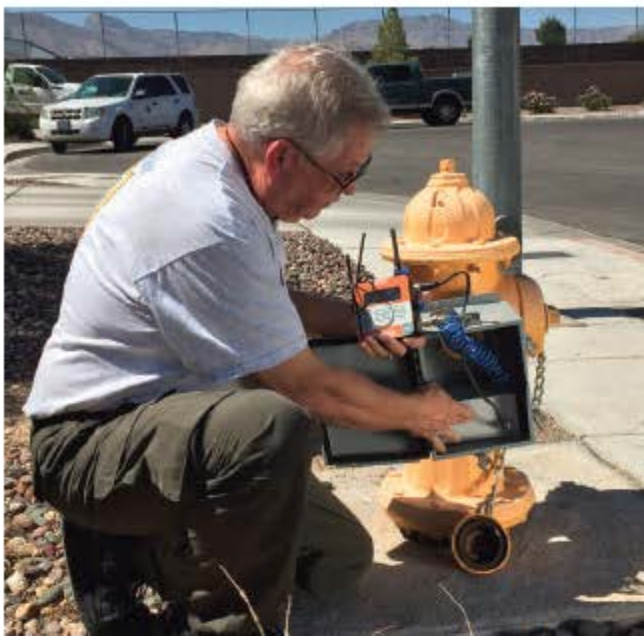
Installed on 1/4" service connections and fire hydrants, the units were configured to monitor continuously at 128 samples per second.
