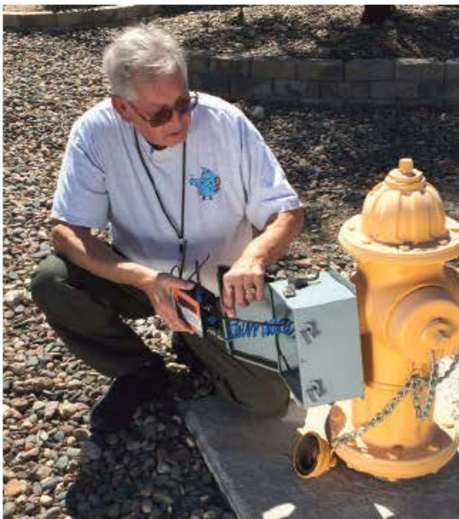
The LVVWD Asset Management Team rotates Syrinix PIPEMINDER units throughout its distribution system.
